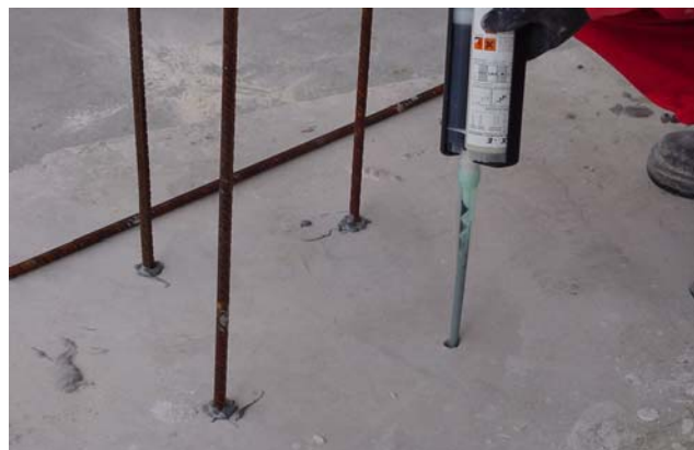
Figure 28.- Anchoring of reinforcing bars on slabs or concrete with MAXFIX ® -E epoxy resin-based injection system
